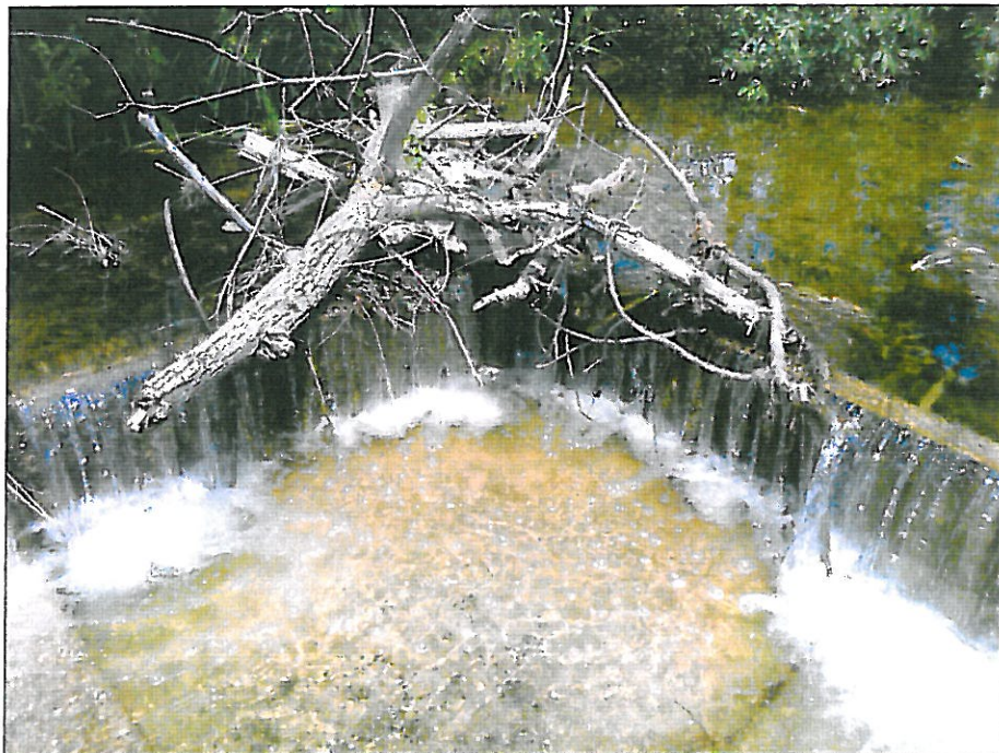
AT DAM LOOKING NORTH TOWARD DEBRIS ON WEIR
